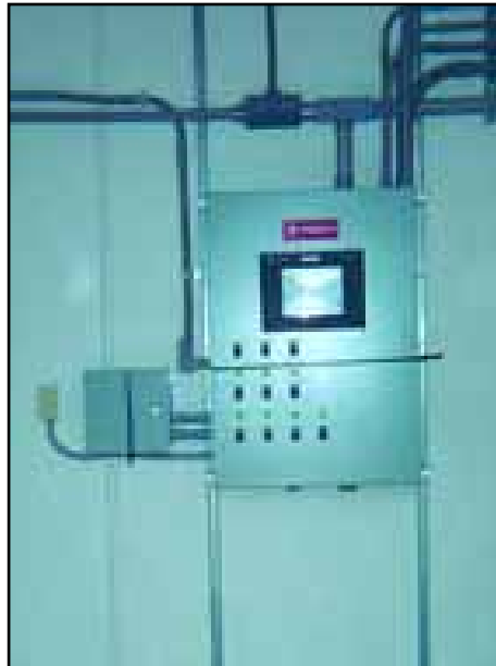
Here shown is the inside of the office and the system Master Control/Telemetry panel. The control panel contains an Allen-Bradley SLC 503 PLC which controls the total process from wells forward to the booster station all based on elevated tank levels. Each well has a PLC based radio telemetry RTU communication with the master control panel shown.
