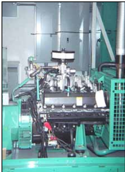
Here shown is the emergency, natural gas engine generator set with an automatic transfer switch and utility power entrance.
