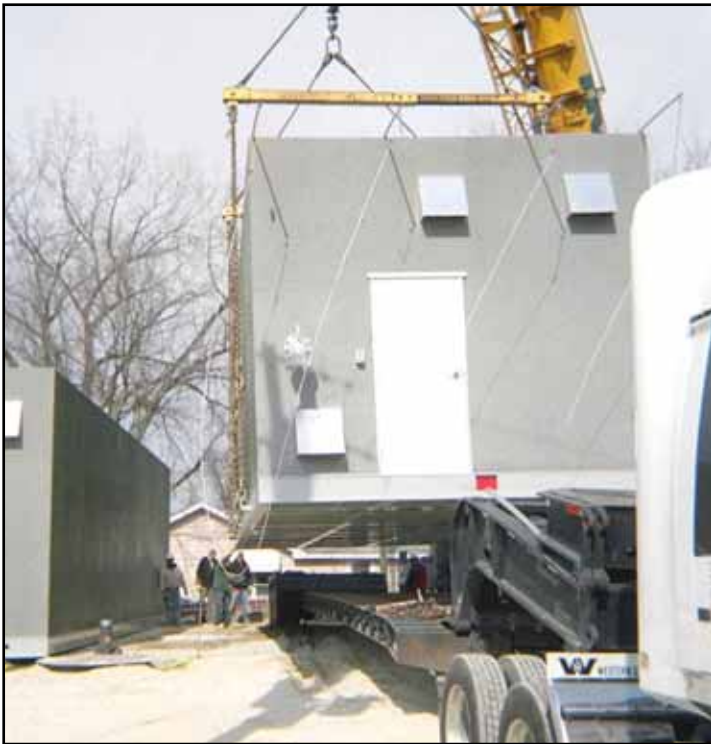
Here shown is the eastern half of the treatment facility being lifted for placement on the foundation next to the western half.
