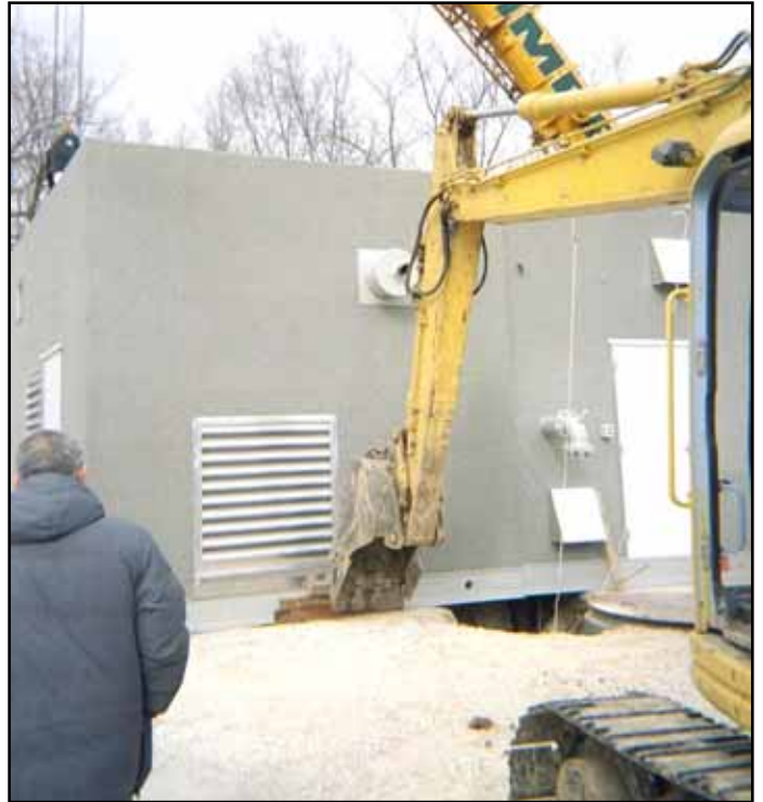
Here shown is the western half being moved into its final position by having the crane lift the back edge slightly while a push is given to the front end by a small backhoe.
