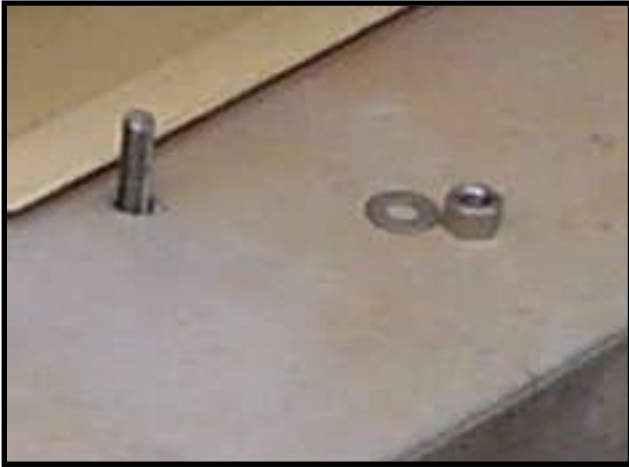
Contractor furnished anchor bolts have been bonded in place with a vinylester-based anchoring adhesive.
