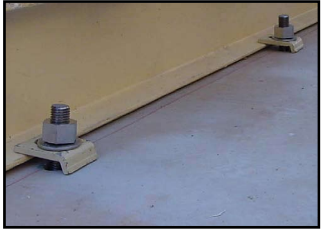
EFI provided anchor clips are installed to anchor the station to the slab.
