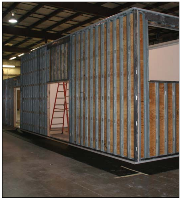
One of the two building halves in fabrication at our factory in Centralia, Illinois.
