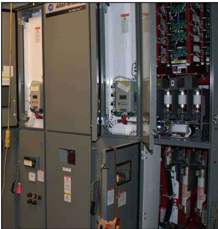
Motor Control Center (4160 Volt) being assembled. Each half of the building had its own set of pumps and controls with separate power feeds for complete redundancy.
