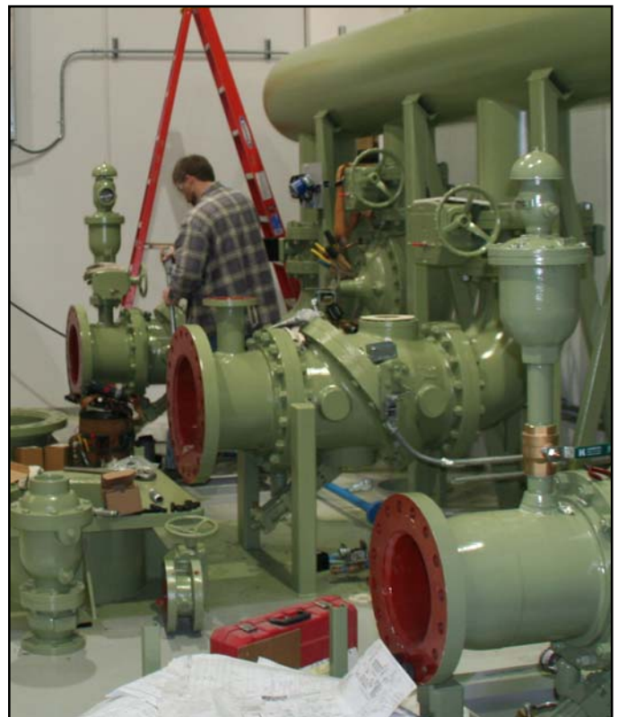
Shop assembly of mechanical components including pump check valves, isolation valves and the discharge header.
