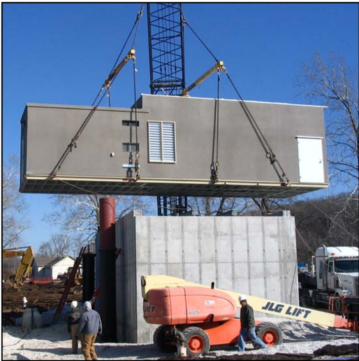
First of two building halves being lifted and placed on top of the intake structure. The low roof portion is the electrical room and is separate from the pump room.
