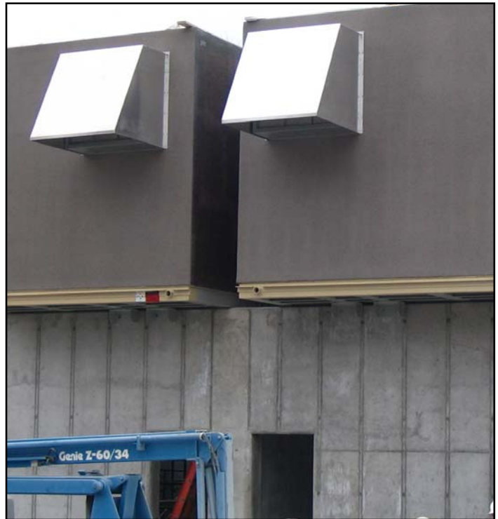
Both building halves being set into place side-by-side with the roofs to be lifted into place later.
