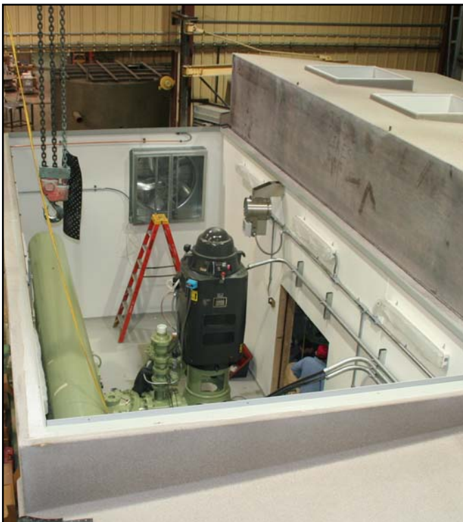
Building halves being assembled on shop floor. The buildings were assembled side-by-side at the factory, and then disassembled for shipping and final installation in the field.
