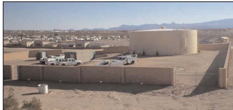
Finished station on start-up day with EFI service truck next to pump station.
