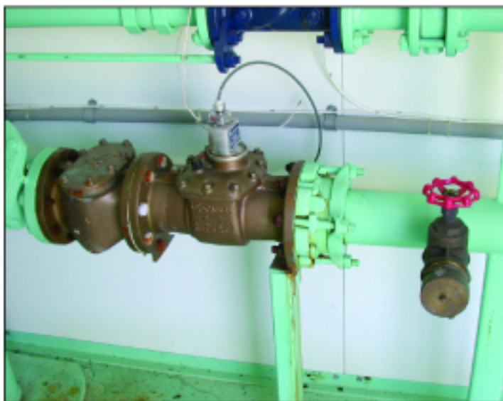
This installation shows a screen attached directly to a 2-inch meter. Down stream from the meter a 2-inch valve is attached so that the meter can be tested in place.
