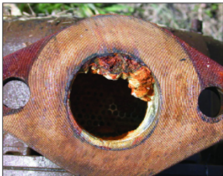
This is what can happen if proper maintenance is not performed regularly on a system's meters. When tested this meter was over registering which led to the water system showing a water loss.
