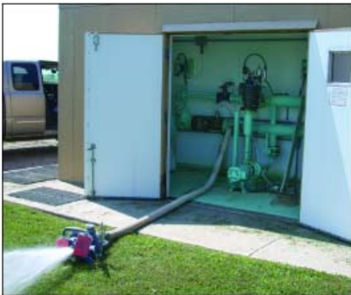
This booster station is set up to allow the master meter to be tested "in place." A test port allows for KRWA's test meter to be placed downstream of the system's master meter with no need to remove the large meter from its normal position.
