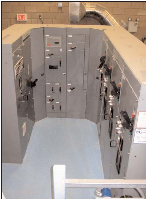
Motor control center.
