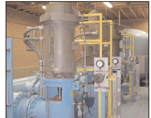
Installed motors and vertical turbine pump heads.
