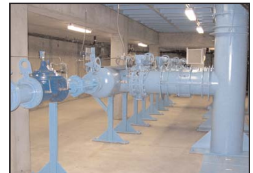
Basement view of piping for the turbine pump barrels.
