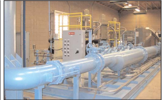
Station installed with a view of the discharge piping.
