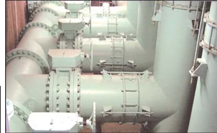
Fabricated steel pump and header piping.
