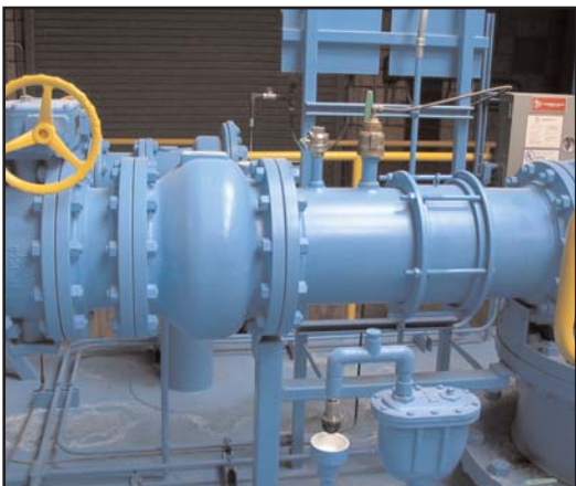
Pump discharge check valve.
