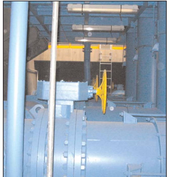
Basement piping gallery suction isolation and pump barrels.
