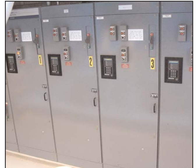
Motor Control Center.
