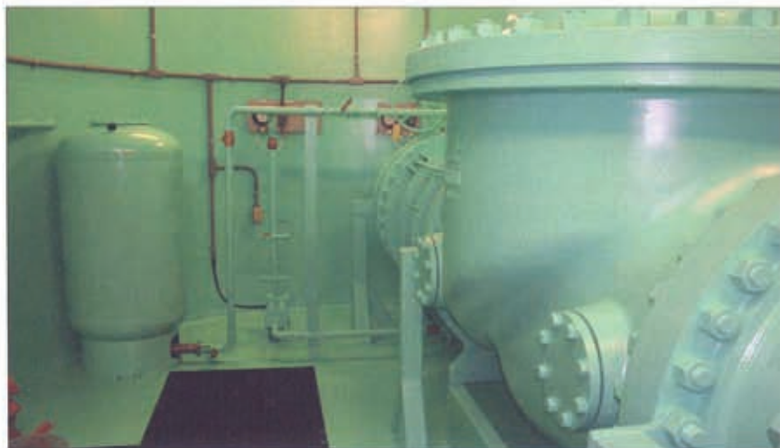
Shown here are the pilot water system tank, pump, and piping. Behind the 36-in. control valve is the breakaway coupling included to facilitate valve withdrawal if ever required.
