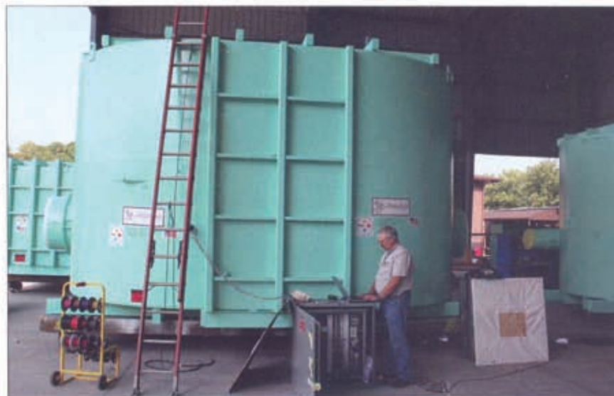
Here, Mike Johnson, one of EFI's Control System Designers/Programmers, exercises the control system and the valve solenoids as part of the final QA checkout.
