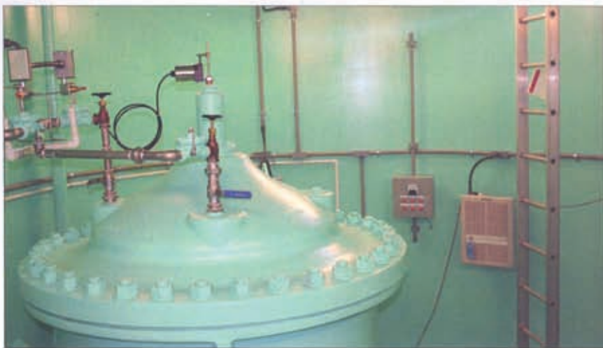
The dome of the valve and the tank wall welding along with the ladder to the manway hatch, the heater, the cathodic protection system, and the anode test station are shown here.
