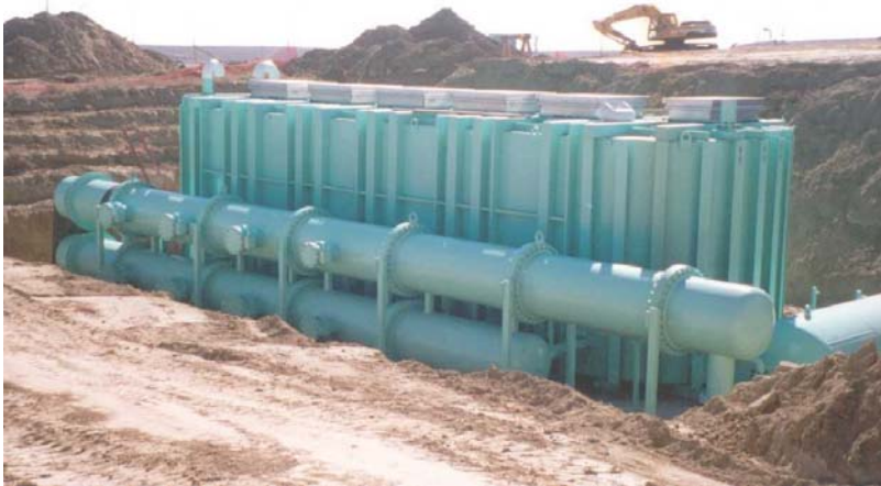
Greeley, Colorado Booster Pump Station
