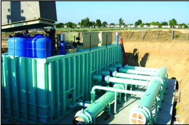
31.6 MGD Booster Station Thornton, Colorado
