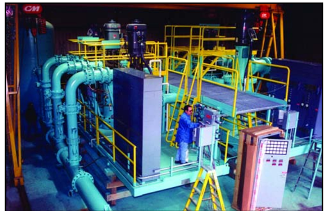
42 MGD Pump Station Henderson, Nevada
