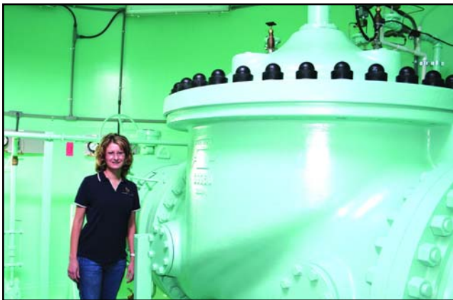
36" Pressure Reducing Valve Station Warren, Michigan
