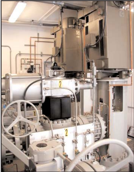
Pumps and discharge control valves for high pressure service.
