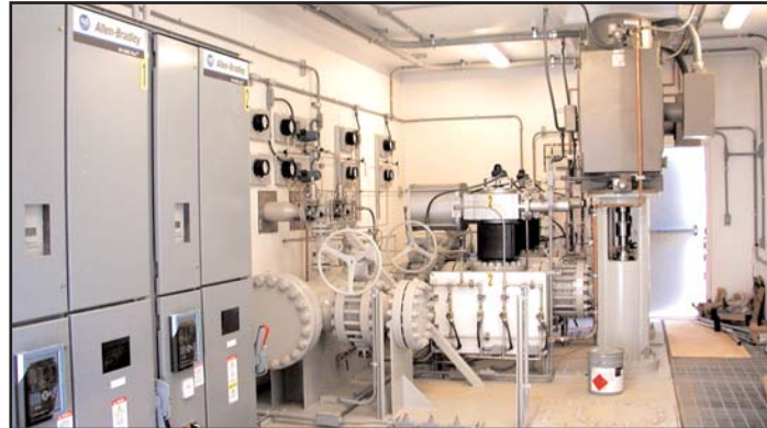
Interior view with pumps set.
