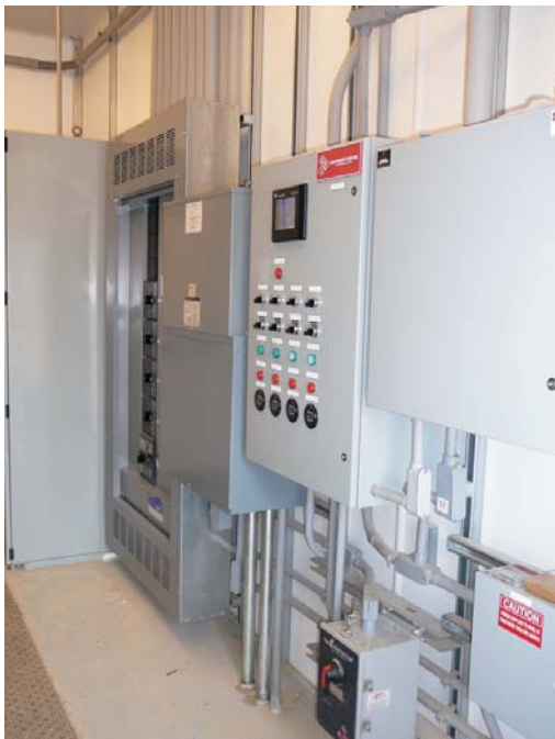
Pump controls and power distribution equipment nearing completion.
