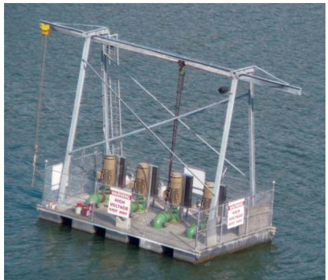
Floating pump barge on Lake Cumberland in Kentucky.
